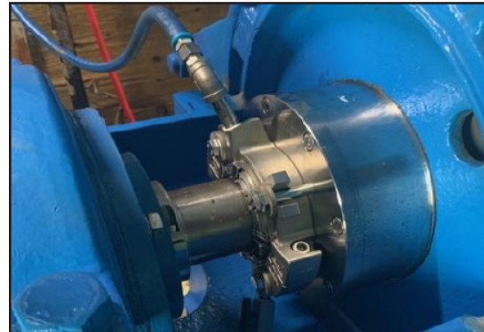
Pump installed with a Chesterton® 442 Split Seal and a SpiralTrac® Environmental Controller.
